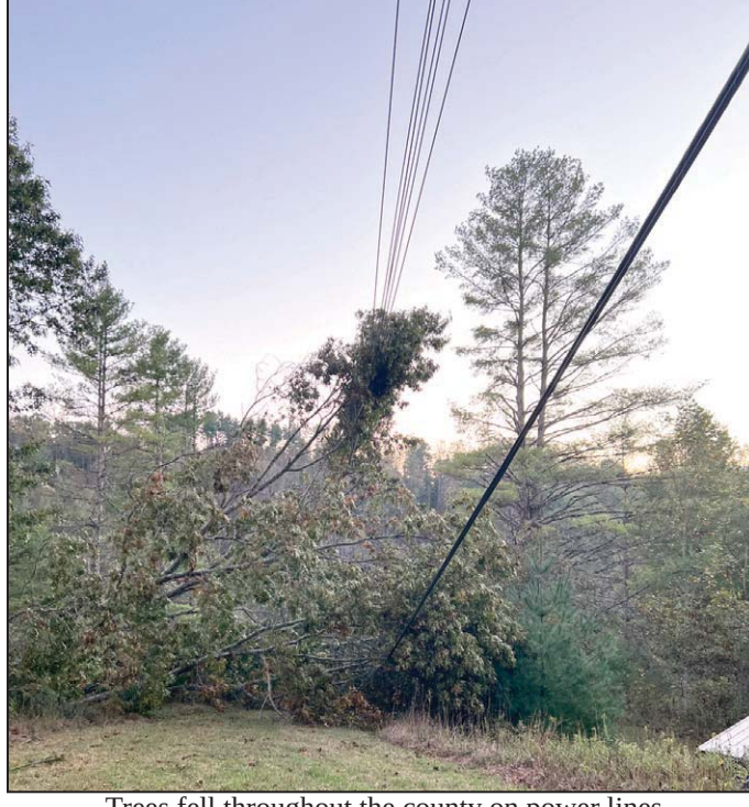
Trees fell throughout the county on power lines
